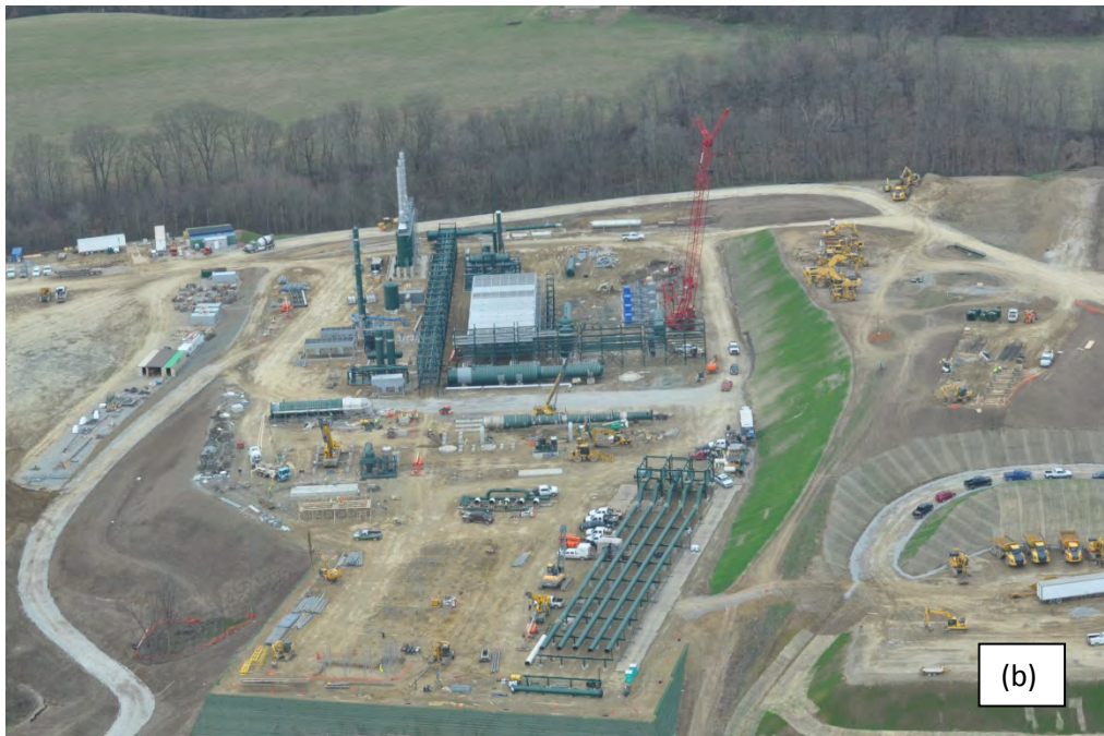
Figure 9. (a) Three Brothers Compressor station in Smith Township. Lat 40;19;40.698. Long 80;23;25.236 (b) New processing plant under construction in Smith Township. Lat 40;25;3.402. Long 80;20;44.951 Photos courtesy of Bob Donnan.
